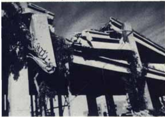
The double-decked section of I-880 in Oakland collapsed, crushing motorists on the lower deck.
