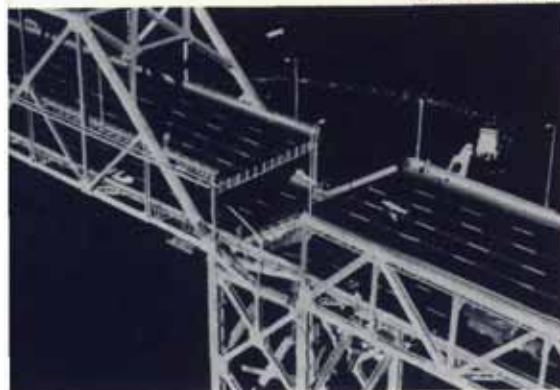
The section of the Bay Bridge upper deck fell when a bridge footing slipped out of place.
