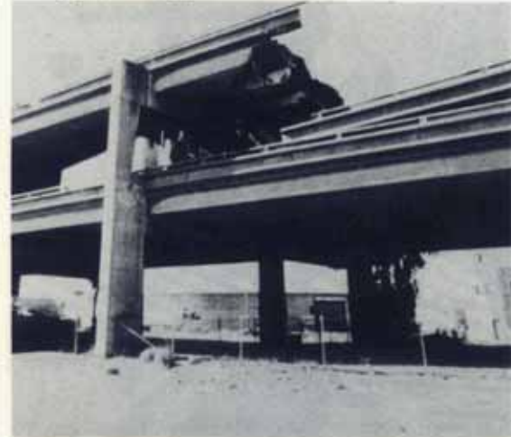
Damaged section of Oakland Cypress structure.
