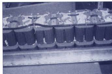
Lots of batteries...
